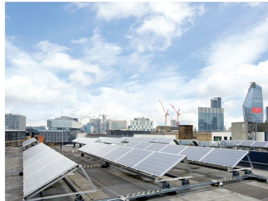
The solar PV panels on the roof of the Metal Box factory were installed in 2015 and have since generated a total of 106,830 kWh. This is a prime example of how older listed buildings can be retrofitted with renewable technologies.
